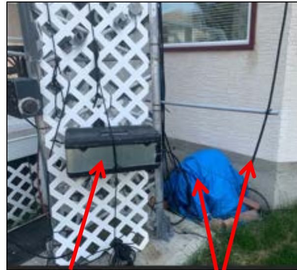
Shunt capacitor and motor
